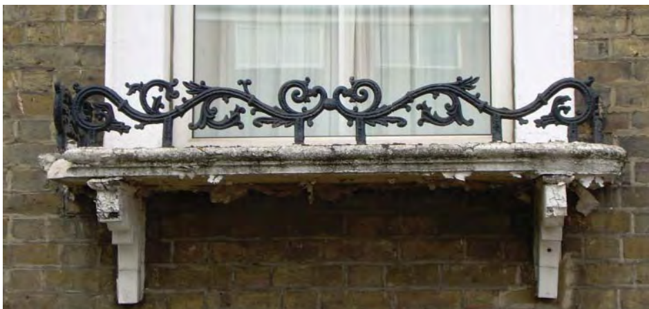
Decorative ironwork window box, an important surviving historic feature although in a poor condition, situated on a projecting timber sill
