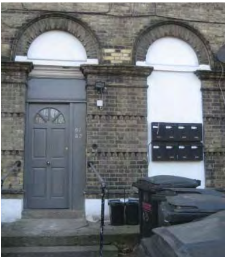
Inappropriate alterations to doorways
