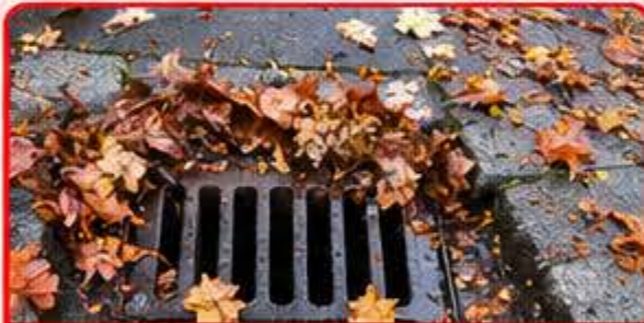
Leaves blocking gullies and drainage causing potential flooding
