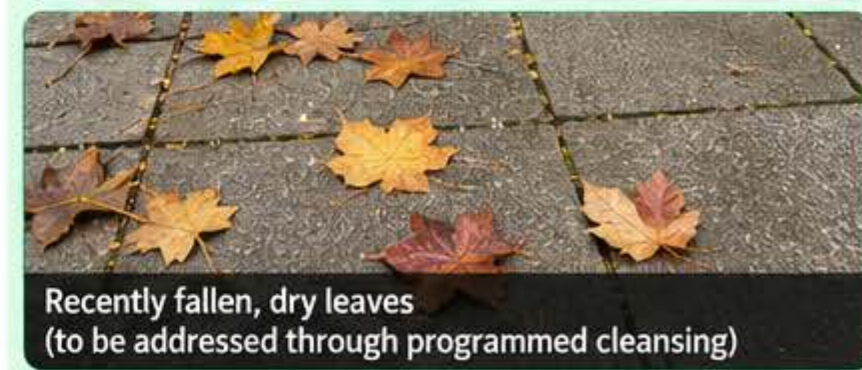
Light scattered leaves on pavement and road (no immediate safety concern)
