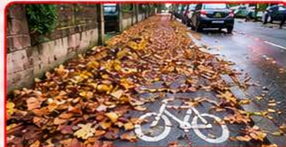
Heavy accumulation blocking cycleway and pedestrian access
