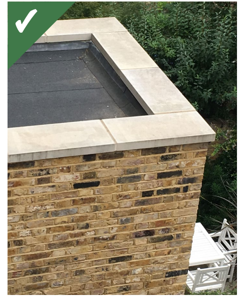
Figure 4.24a: A parapet can be used on a flat roof to remove the need for gutters, creating a less cluttered appearance.
